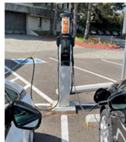
Single pedestal EVSE serving three spaces including an ADA-compliant space. WSDOT, Shoreline (Photo: WSU)
