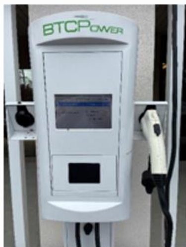
Dual-port wall-mount unit attached to a building column. Shows L2 J1772 plug. Dept. of Commerce, Olympia (Photo: WSU)
