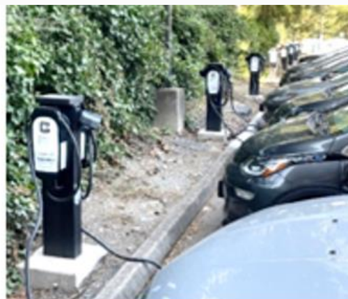
Dual-port L2 EVSE set apart to charge EVs side by side. In-ground conduit to individual concrete pads.
