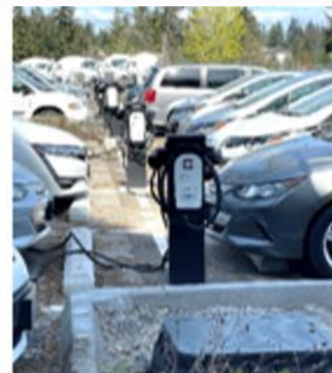
Utility box in foreground serves L2 EVSE in a row for EVs on both sides.
